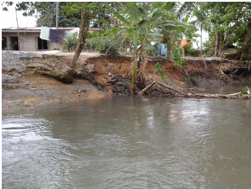
Fig. (9): Failed sections of River Bank due to accelerated erosion
