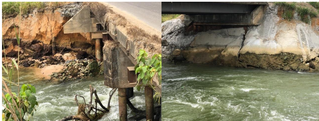
Fig. (5): Akpajo Bridge abutment deterioration Upstream Reach Okpoka River
