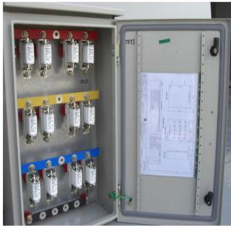
Plate 1. 4-Way LT Feeder Pillar
