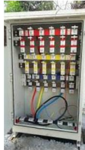
Plate 2. 6-Way LT Feeder Pillar
