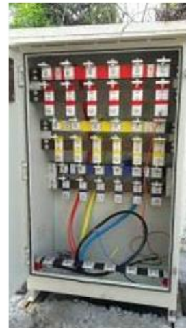
Plate 2. 6-Way LT Feeder Pillar
