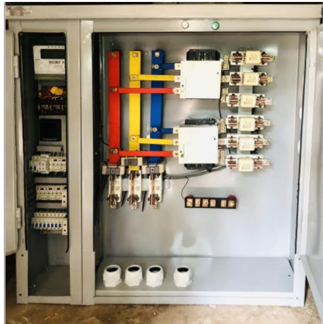
Plate 6: The inside of Novel Electricity Distribution Pillar (open)
