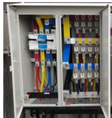
Plate 4. 4-Way LT Feeder Pillar with Manual Switchgear
